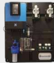
CONTROL STATION PANEL
